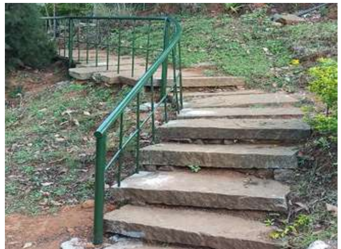
The roof of one of our campus buildings (above) and the railing of a pathway (below) after repair work - these are some of the several improvements made to the campus infrastructure this year.
