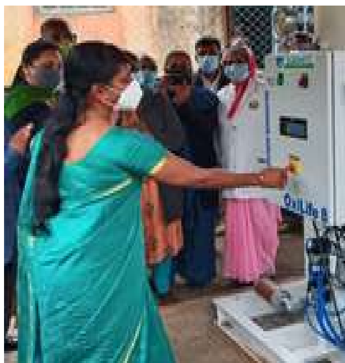
Keystone enabled the installation of oxygen plants during the COVID-19 pandemic.
